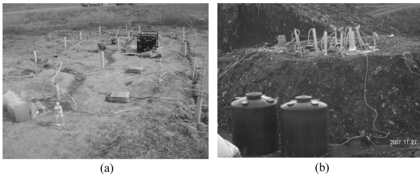
Figure 8. Details of electrokinetic reactive pile experimental setup. (a) Field installation of electrokinetic reactive pile system for remediation of in-situ soil; (b) Field installation of electrokinetic reactive pile system for remediation of sorted soil.
